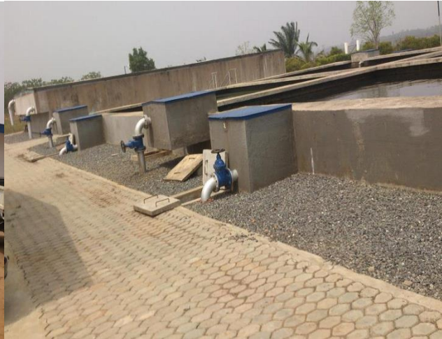
3-District Water Treatment Centre at Aveyime
